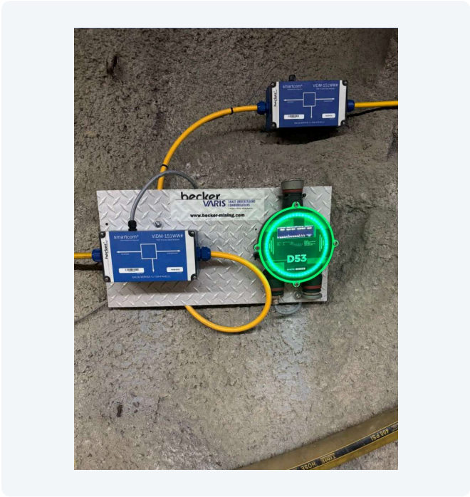
Example field installation for fixed-area monitoring.
